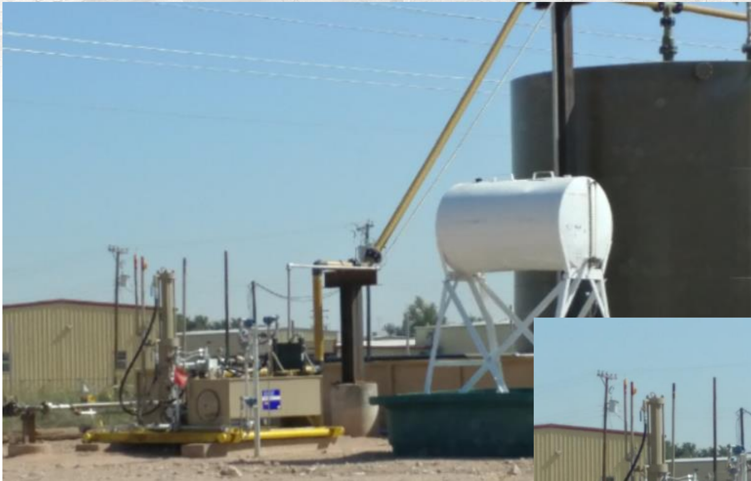
Vapor Recovery Unit 16% H 2 S
