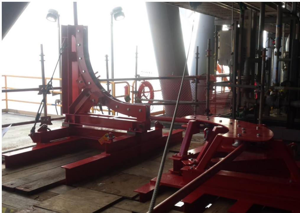
2 – Roller Sheave's (lower deck)
